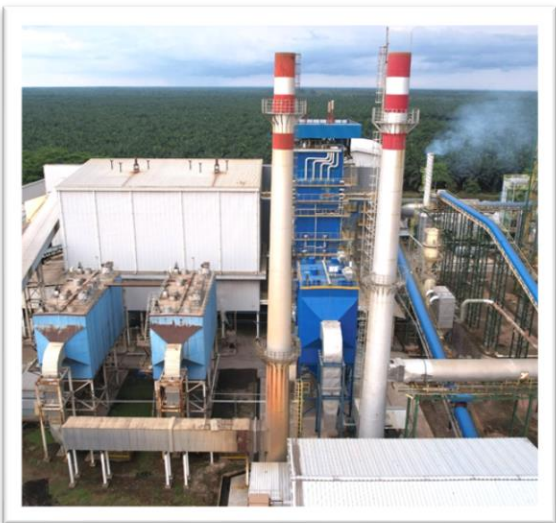
POWER PLANT Capacity : 30 MW Turbine, 2 Boiler x 40 ton & 1 CFB Boiler x 80 ton
