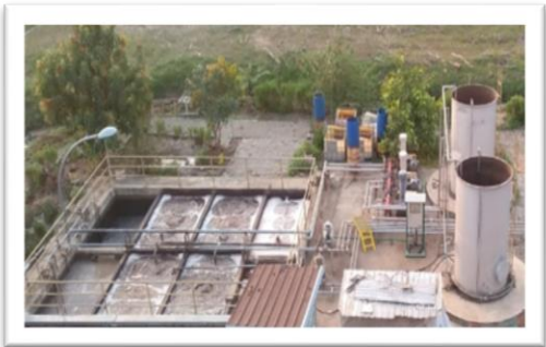
WASTEWATER TREATMENT PLANT
